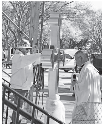
Father Jeremy Secrist blesses with holy water the new steeple cross at St. Peter Church in Jefferson City before it is lifted into place on March 29.
